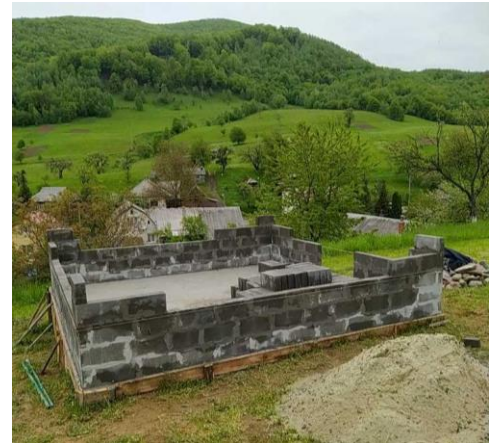
Building a place for chickens to help grow food in the village in Ukraine.
